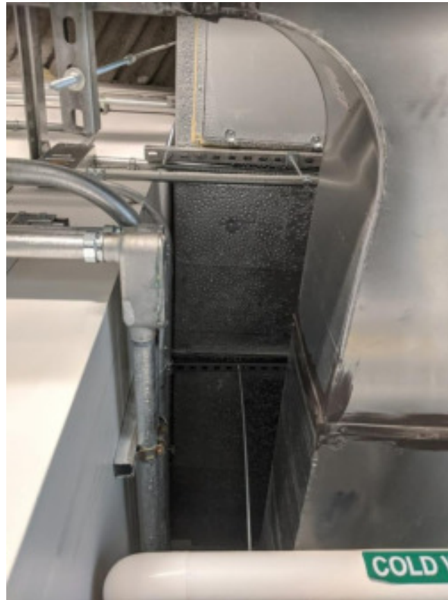
Figure 2: Facility Walk-Through Photo
